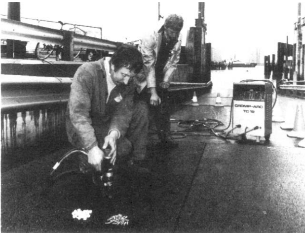
Figure 19.4 A Crompt-Arc TC12 electronic welding system being used to install a new anti-skid surface at a ferry terminal (Crompton Parkinson)
