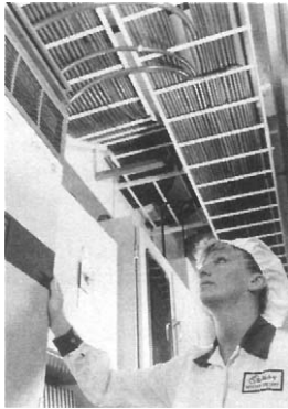
Figure 22.10 KHZ hot-dip galvanized cable ladder having oval rungs and closed rail profile meets Cadbury's stringent requirements at its Bournville factory (Wibe)
